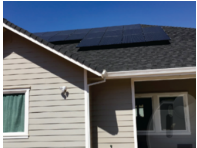
5.3 kW Solar PV
