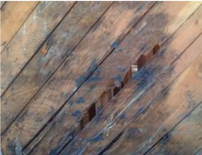
Exterior walls moisture damage
