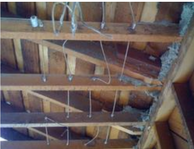
Attic: knob & tube, no insulation
