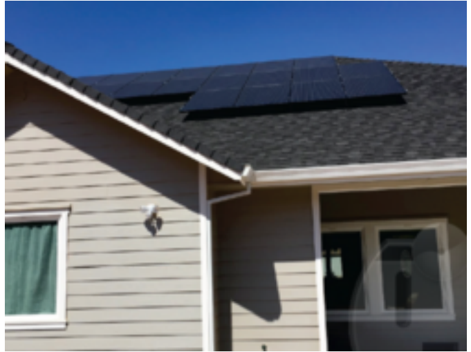
5.3 kW Solar PV
