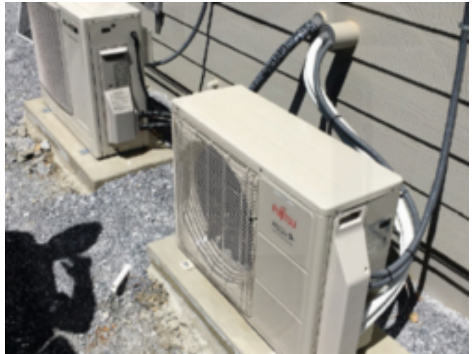
Fujitsu 3/4 ton mini-split heat pump: heating & cooling
